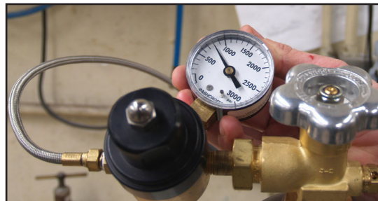
Fig. 33 Source tank pressure gauge
